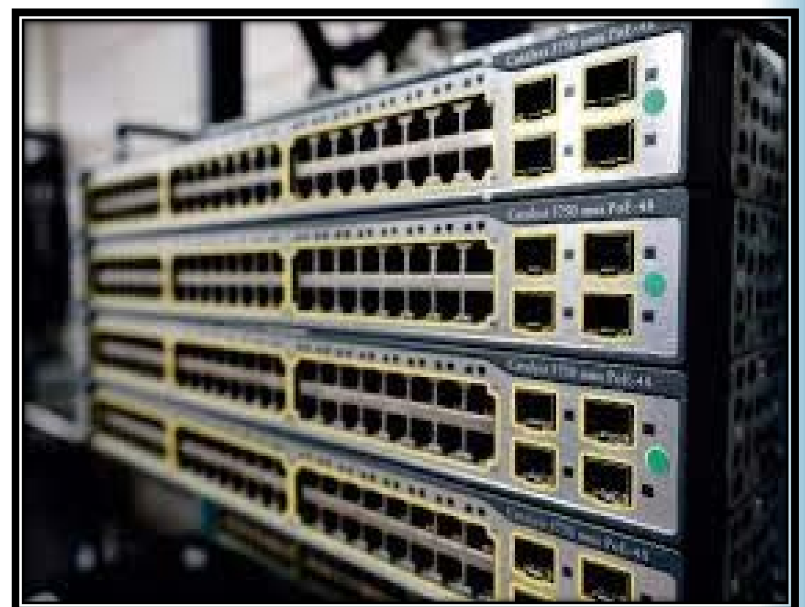
Systemwide I.T. Switch Replacement Project
