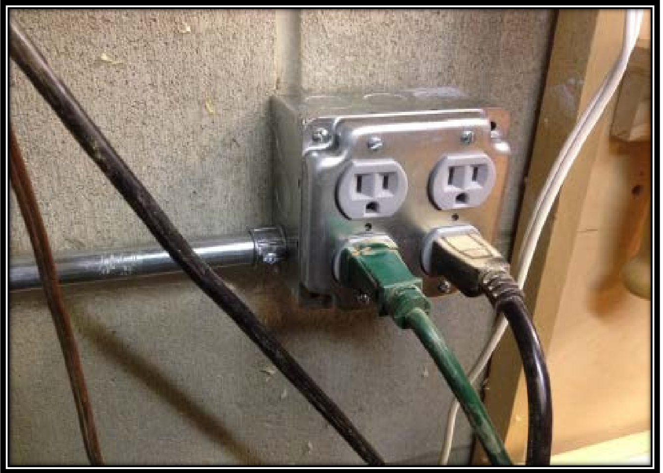
Electrical power quad outlet
