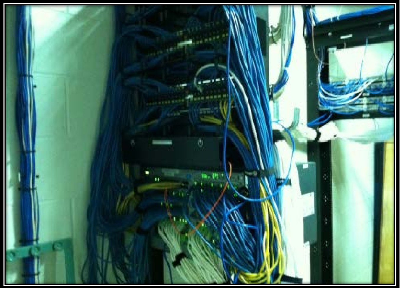
CAT 6 low voltage rack cabinet
