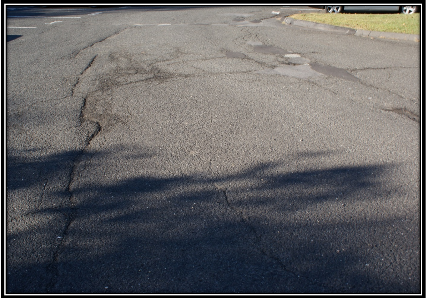
FLHS student parking lot deterioration after more than 13 years of use
